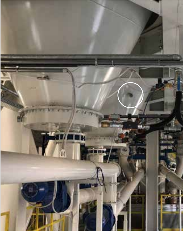
VBS (aireadores) - Silos
